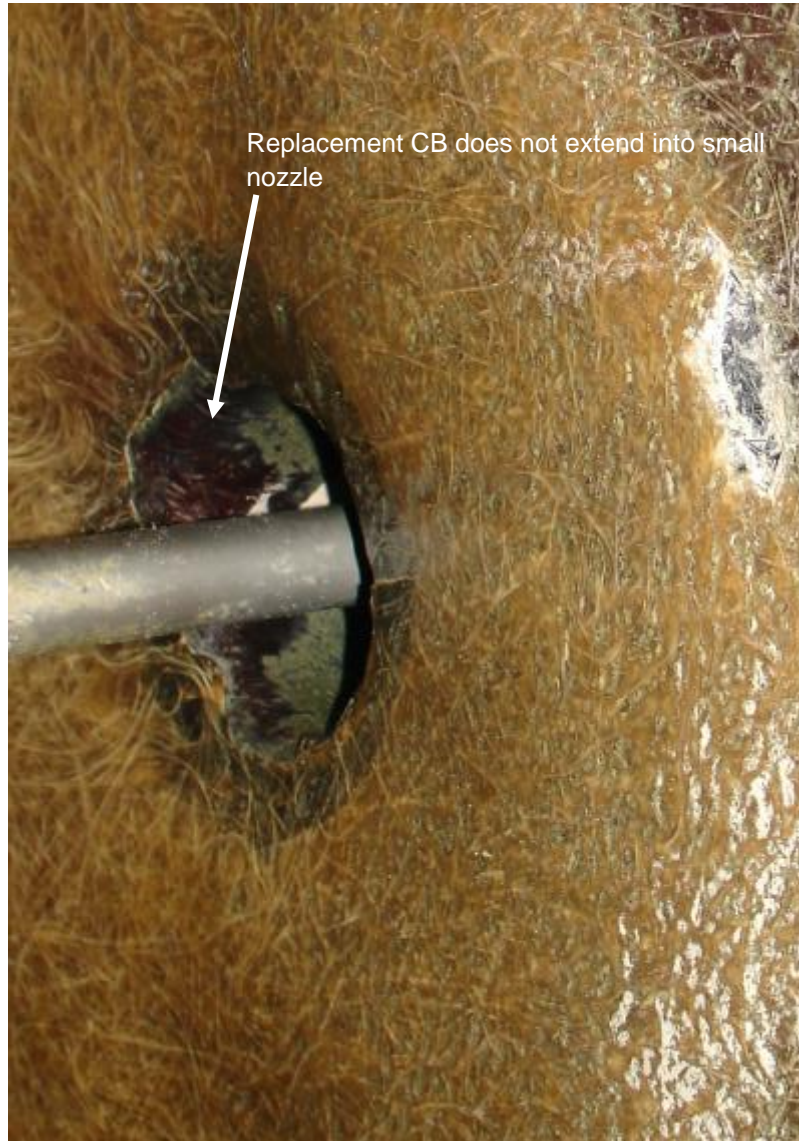
Figure 5 – Current relining at small bore nozzles
