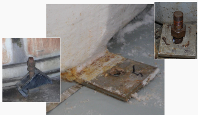
Figure 5. Anchors and hold-downs that require corrective action.
