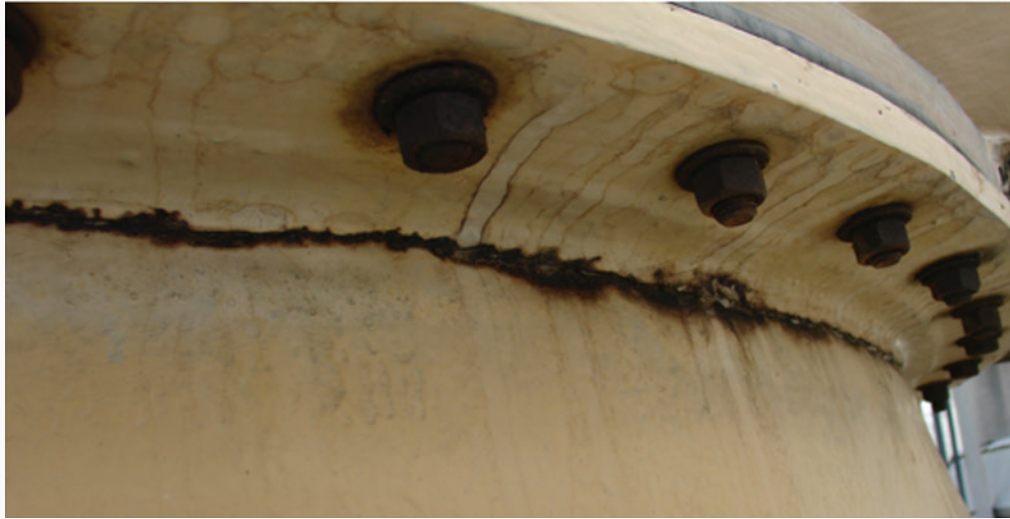
Figure 9. Body flange where corrective action is required.
