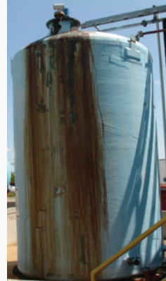
Figure 13. Tank with no overflow; corrective action is required. Note the staining from overfill spills out of the top nozzle. While this tank has not yet failed, every overfilling event creates a new risk of failure.
