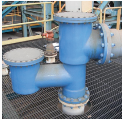
Figure 14. Combined vacuum breaker and pressure relief. Operation can be verified by confirming that the internal disks lift.
