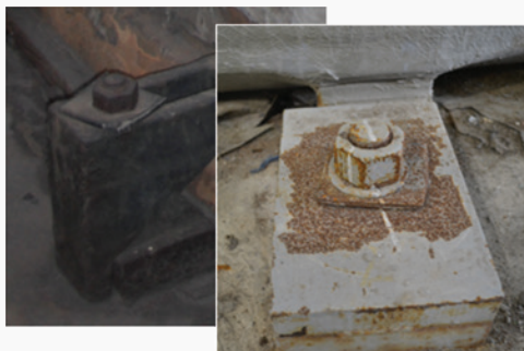
Figure 4. Anchors and hold-downs that do not require corrective action.
