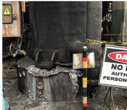
Figure 3. Support that requires corrective action.
