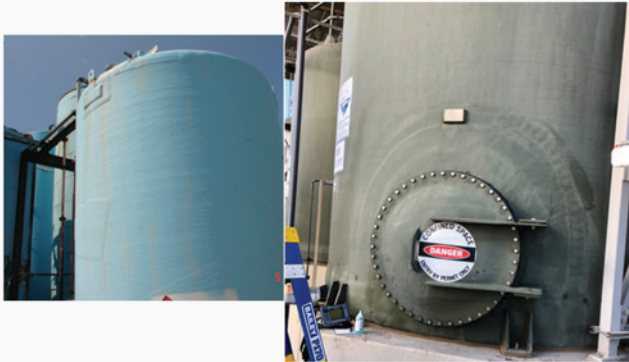
Figure 6. Intact FRP surfaces where no corrective action is required. Note that flaking of paint from the outer surface is normally considered to be superficial.
