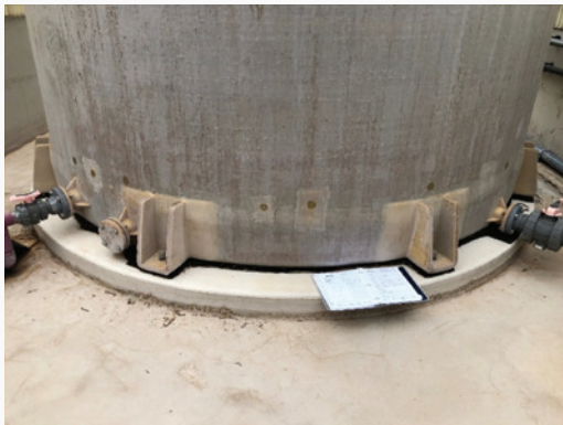
Figure 2. Support that does not require corrective action.
