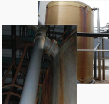
Figure 12. Overflows where no corrective action is required.
