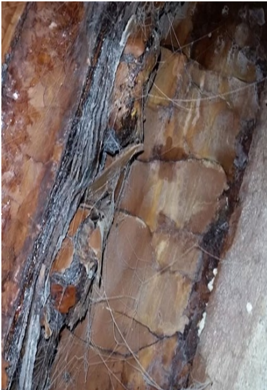
Figure 1 Corrosion of exposed steel
