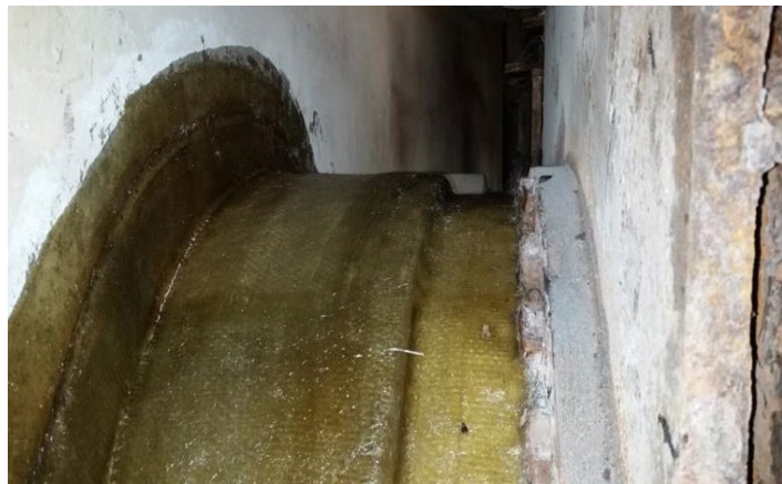
Figure 3 First stage has been applied. When cured, this stage provides a sound surface over pipe and concrete to support lamination
