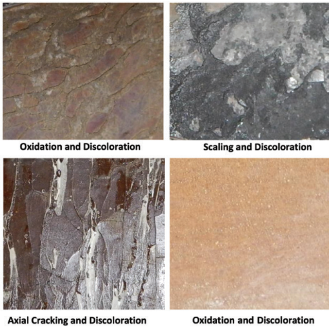
Figure 2. Examples of Corrosion Barrier Appearance
